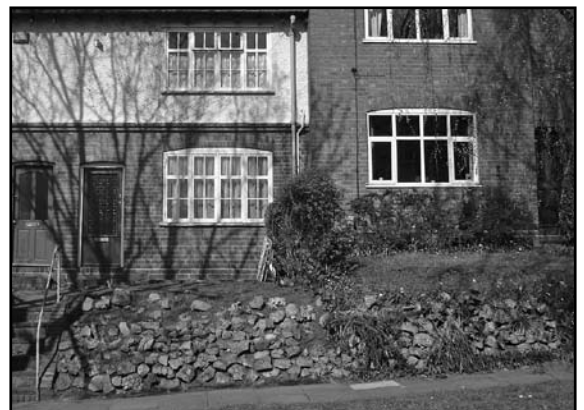
Partially ruined wall.
