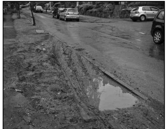
Eroded verge, Margaret Grove.
